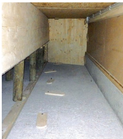
24 Air intake channel
